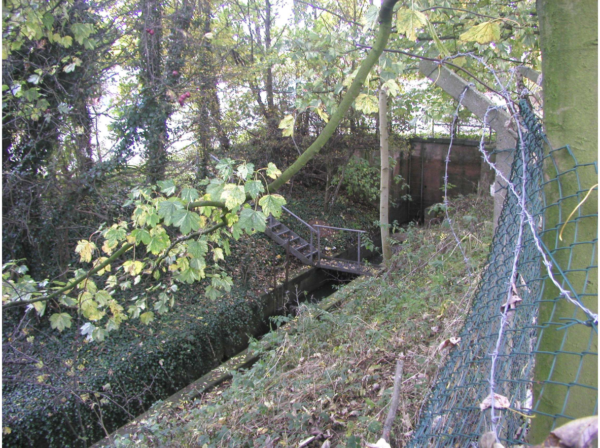
Photo 5: View south west into open channel. Trees by concrete structures need removing to prevent further root damage.
